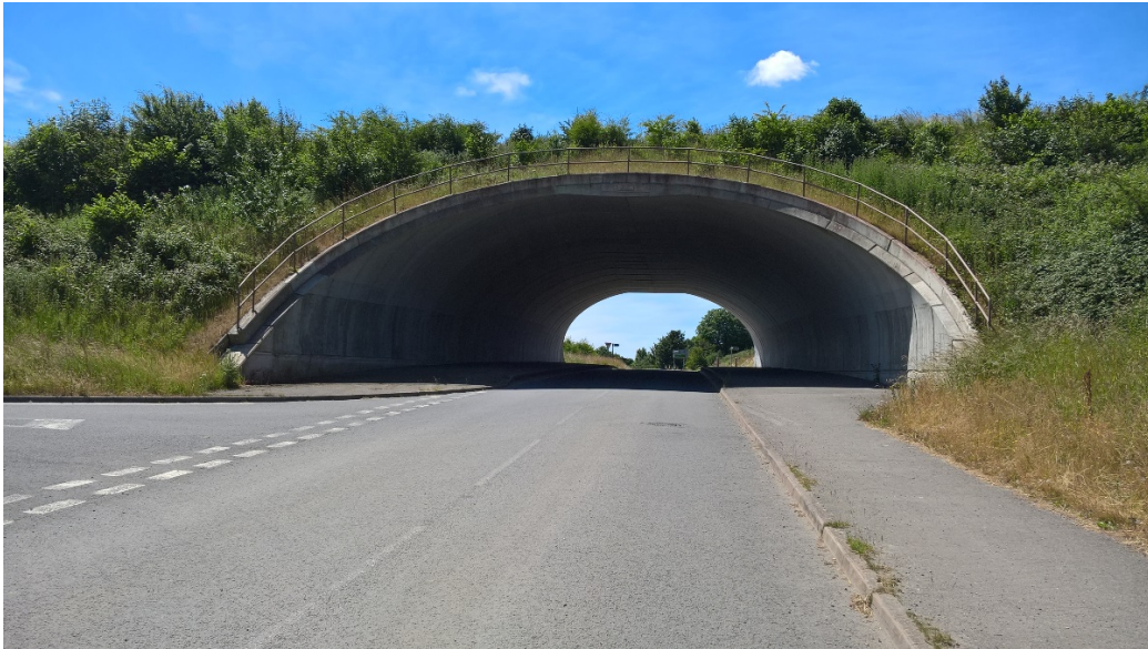
Approach to underpass bridge with dual carriage above, Weymouth relief road scheme
