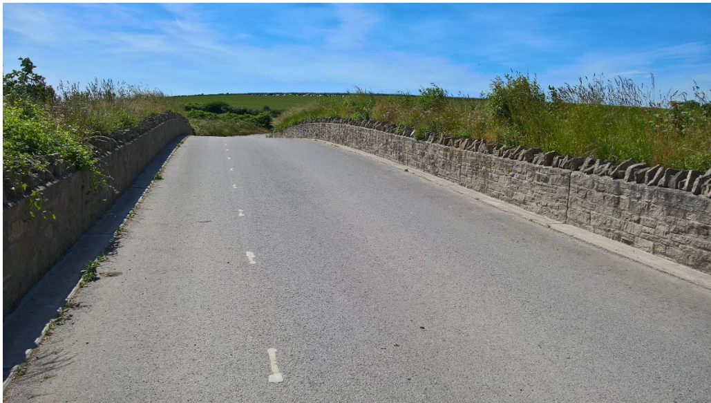
Standing on the overbridge spanning the dual carriageway, Weymouth relief road scheme
